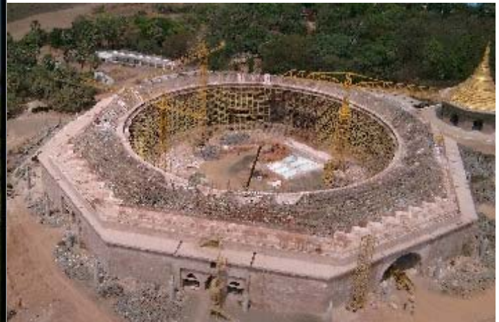
Construction of Global Pagoda, as of June, 2005. The completed small Pagoda (the size of Dhamma Giri Pagoda) is on top
